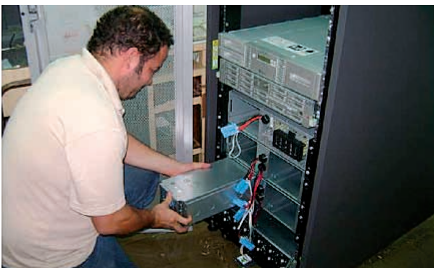
System installation at the NDC of the Dominican Republic, May 2009.
