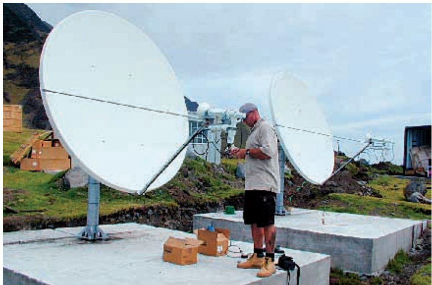
VSATs under construction and (on the facing page) after completion on Tristan da Cunha (United Kingdom), the site of infrasound station IS49 and radionuclide noble gas station RN66.
