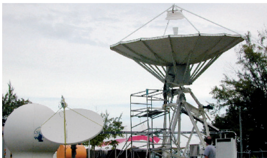
Global Communications Infrastructure VSAT antenna (small dish) relaying data via satellite from hydroacoustic station HA8, located on Diego Garcia in the Chagos Archipelago (United Kingdom), to the International Data Centre in Vienna.
