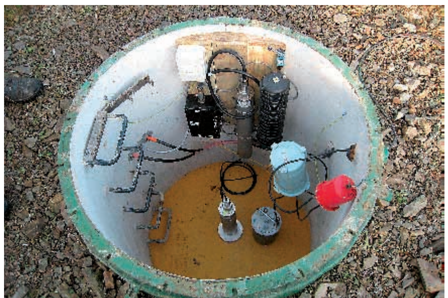
One of the instrument pits forming the seismic array of auxiliary seismic station AS104, Eskdalemuir, United Kingdom.
