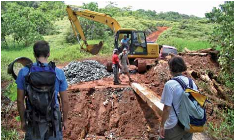
CERTIFICATION TEAM USING U-BEAM TO ACCESS INFRASOUND SITE WHILE BRIDGE IS BEING RECONSTRUCTED, PALAU, JUNE 2005
