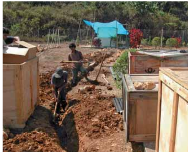
DIGGING A TRENCH FROM THE SENSORS TO THE CENTRAL RECORDING FACILITY, AUXILIARY SEISMIC STATION AS44, KAPPANG, INDONESIA
