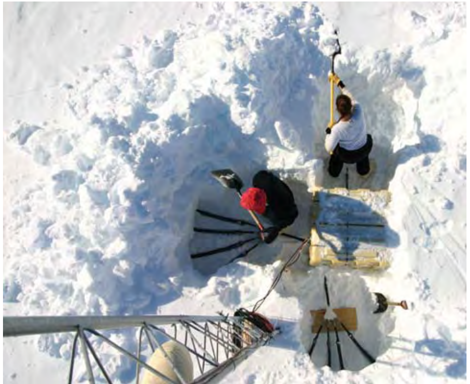
DIGGING OUT THE WIND NOISE REDUCING PIPE ARRAY AND EQUIPMENT VAULTS AT IS55. PHOTO COURTESY OF DUNCAN MARRIOTT, GEOPHYSICAL INSTITUTE, UNIVERSITY OF ALASKA, FAIRBANKS.
