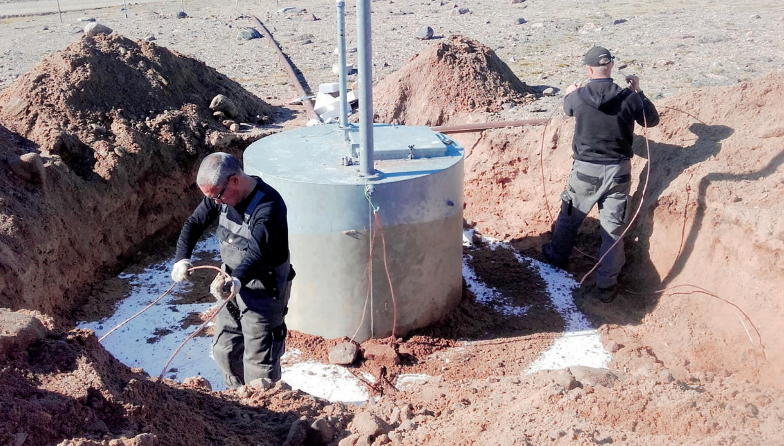
Infrasound station IS18, Qaanaaq, Greenland (Denmark).
