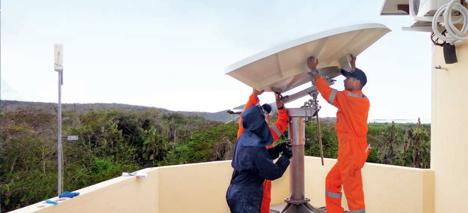
Installation of VSAT equipment at radionuclide station RN24, Isla Santa Cruz, Galápagos Islands (Ecuador).
