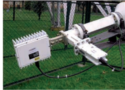
VSAT frequency conversion units for connection to the satellite.
